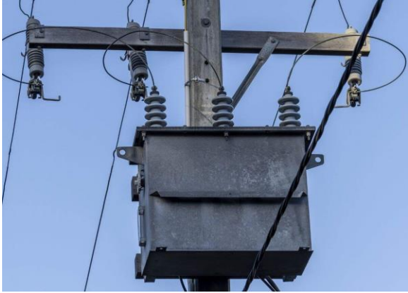
Point of Supply (Transformer, Pillar, Plinth, Pit)
