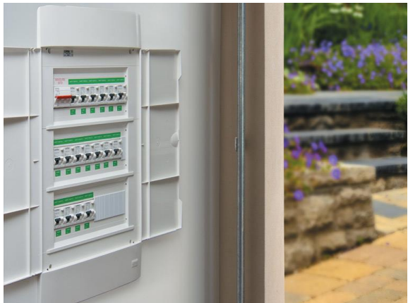
Commercial Distribution Board
